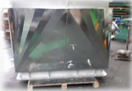
( T/C Outlet Insulation )
